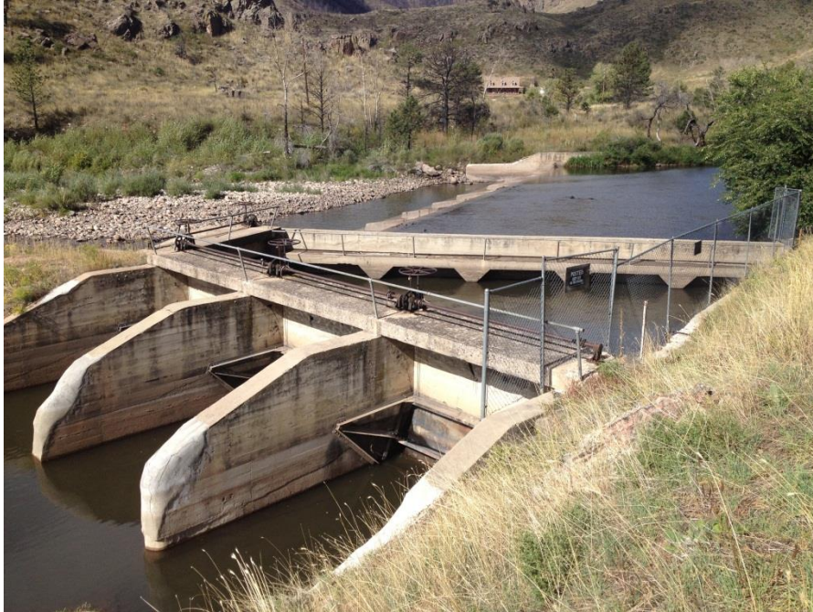
Figure 6. Existing Poudre Valley Canal Diversion on Poudre River near Canyon Mouth
